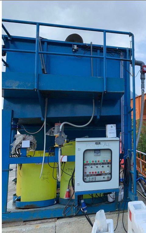
Q1. Wastewater treatment facility 30 cu.m Sedimentation Tank + AquaSed of 15 cu.m per hour + WETSEP
